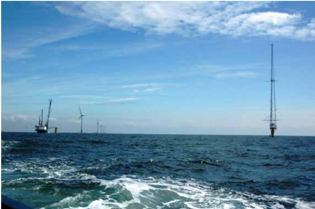
Offshore wind farm Egmond aan Zee during installation, including meteomast near wind turbines 7 and 8. (© J. Beurskens)
